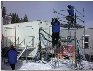
Figure 2.79 Besides more equipment, remotes also take more people. These people must know not only how to operate the equipment, but also how to assemble it into whatever topology is needed to fulfill the client's needs. Here, microwave receive gear is installed on a small scaffold. (Source: Jason Taubman)
